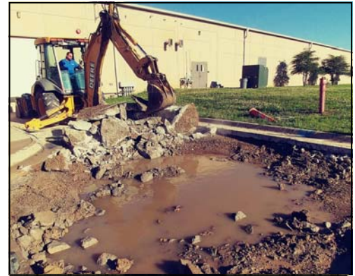
Water main break outside FS Warehouse June 6-8. Mike Brown, Peter Bridges, Dave Bakarich
